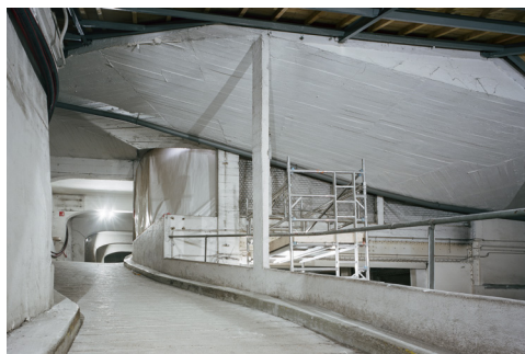
013 Fondation HCB, 79 rue des Archives, February 2017 Vehicle access ramp to the upper levels of the old car park that was destroyed at the request of the architects of Les Bâtiments de France to recreate the 18th century courtyard. © Cyrille Weiner
